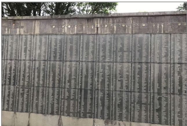
The Memorial Wall before - dirty and rusted.
