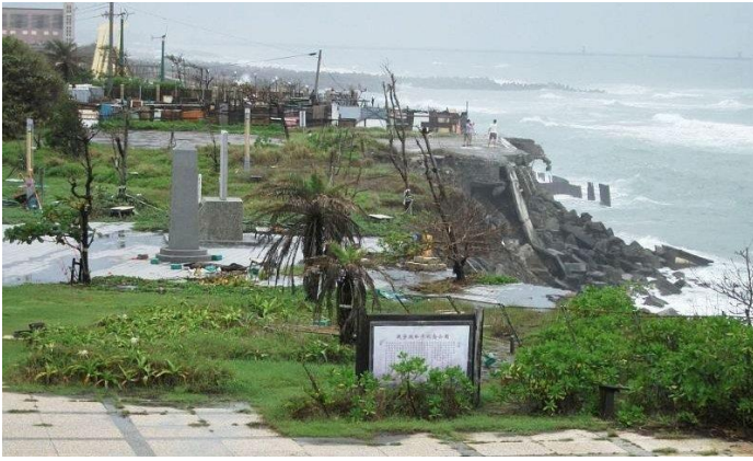
Above: 2012 Photo showing extensive erosion damage to the coastline at the back of the War & Peace Park, which was endangering the memorials.
